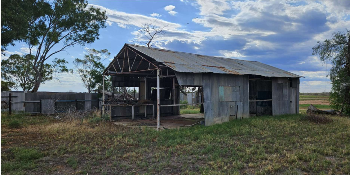
Figure 4: Current dilapidated metal shed that needs to be removed from 100 Hood Street, Wilcannia.
