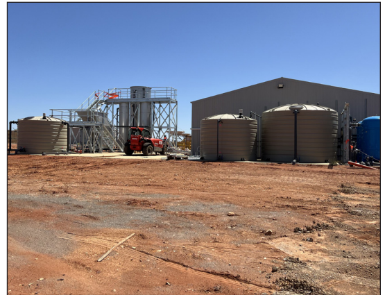
The White Cliffs Water Treatment Plant is expected to be completed in November. Work started in March this year. The Reticulation works at White Cliffs are also progressing well and almost finished.
